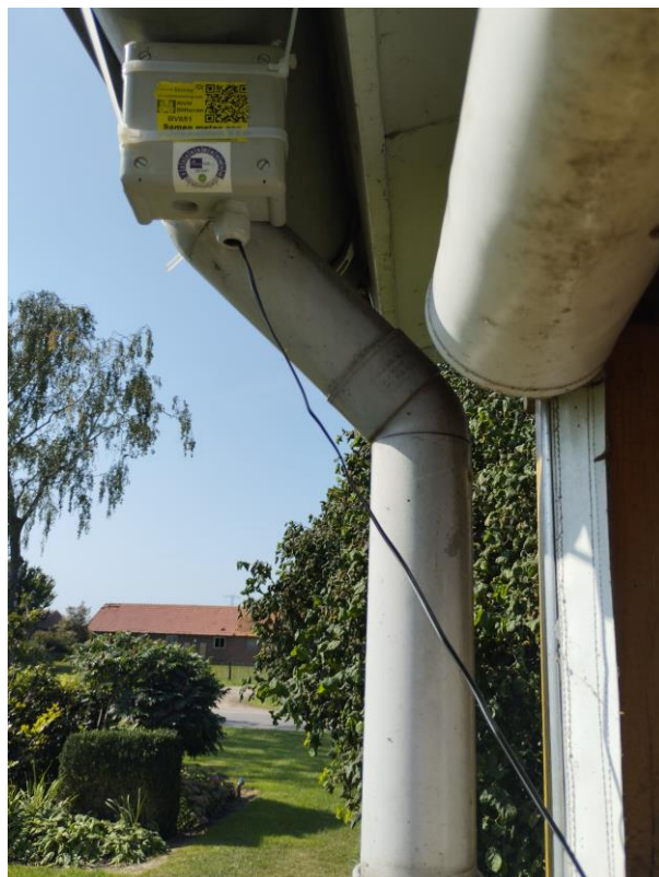
Fig.4: Example placement of a PM10 measuring sensor
